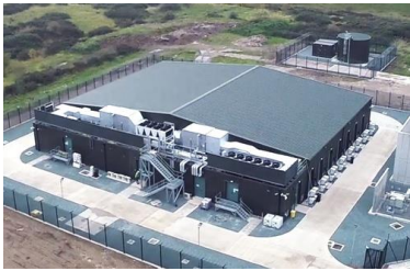
1 Battery 50 MW in Roosecote, UK
